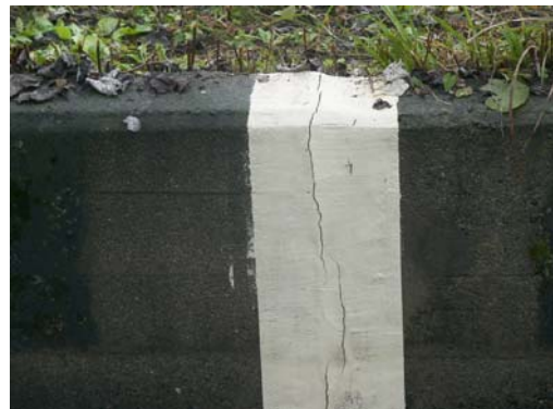
Fig.2 既往の目地補修工法の早期ひび割れ Crack observed at early stage after over-coated repair
